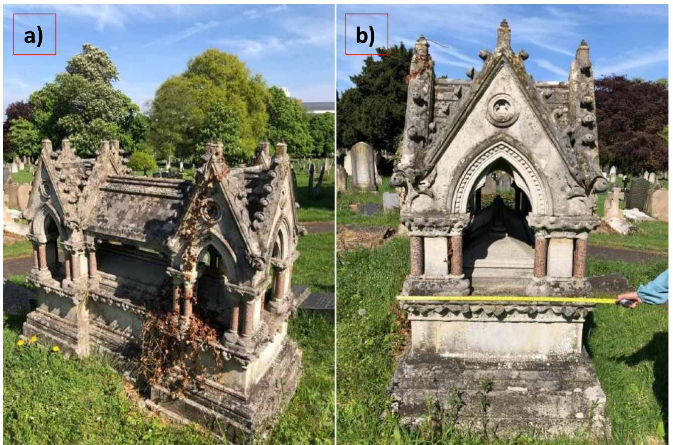
Figure 6: The two merged images (a) show the site where the monument is located ; (b) shows the monument being manually assessed prior to SfM photogrammetry using tape measure.
